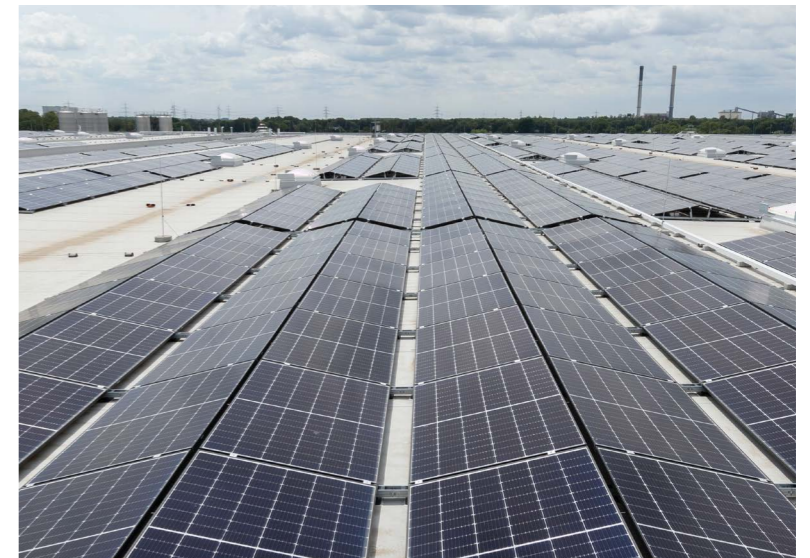
Large-scale PV system for electricity generation
